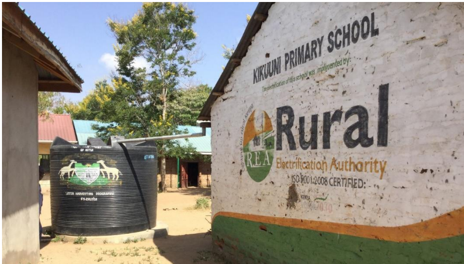
Picture 3.8: Rainwater harvest and storage systems installed in Kikuuni Primary School to address the perennial water shortages
